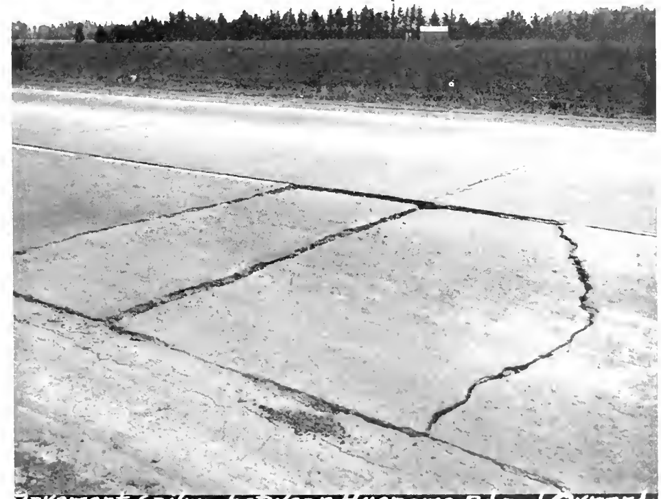
Pavement failure between Hueneme Rd and Oxnard
